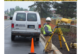
Land Surveying is completed with GPS and Robotics for efficient and accurate surveys used by the engineers
